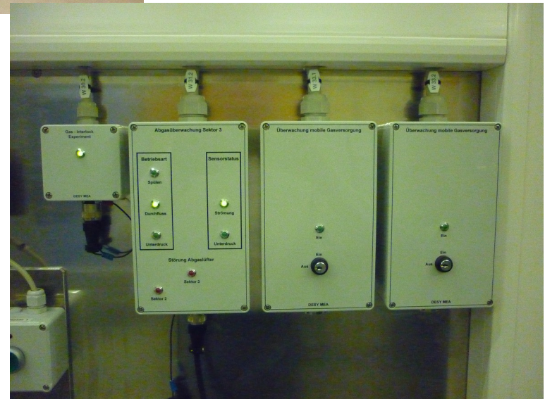
Safety system for sensors and exhaust control
