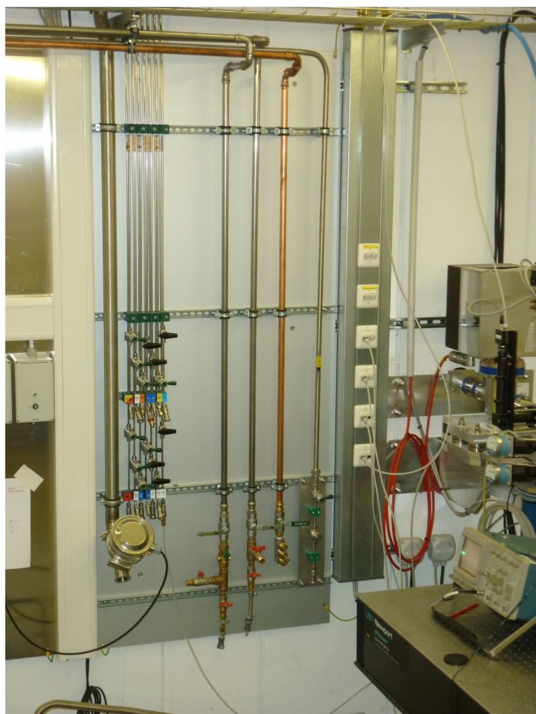
Gas connectors, pressurised air and cooling water at P65
